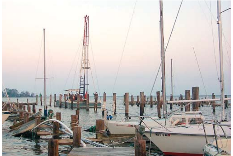
A storm surge during Hurricane Isabel combined with normal high tides to overcome this low-lying breakwater. The protected harbor then became an open bay and many of the boats in the harbor either sank or were badly damaged.
